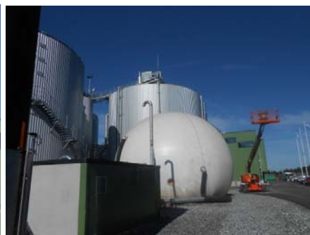
Biogas collection tank
