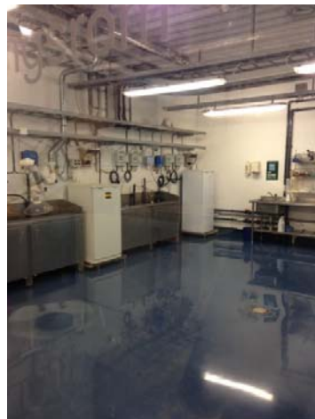
Inline testing and auto sampling
